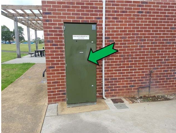
Photo 1. Exterior, north elevation, electrical backing board – suspected non asbestos-containing bituminous backing board.
