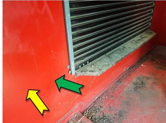
Photo 2. Interior, south elevation, wall – non asbestos-containing fibre cement sheeting and suspected lead-containing red upper paint systems.
