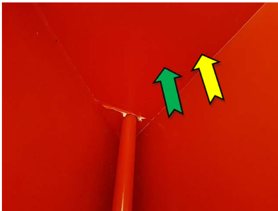
Photo 3. Interior, throughout, ceiling – assumed non asbestos-containing fibre cement sheeting and suspected lead-containing red upper paint system.
