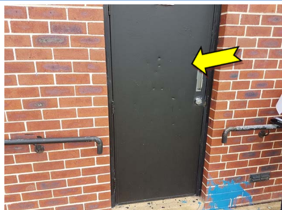
Photo 6. Exterior, east elevation, door – suspected lead-containing black upper paint system.
